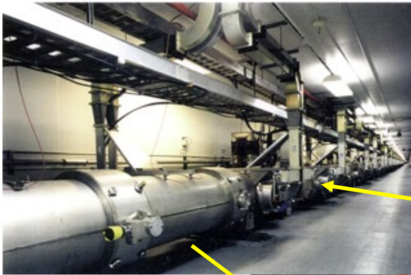
Cryomodules in the accelerator tunnel
