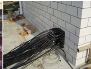
Figure 7. (Right) Photograph showing the 36 main feeder cables running to the main array.
