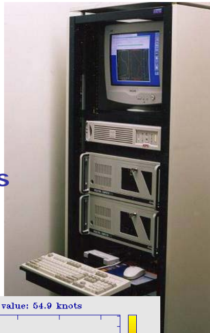
Radar Equipment Rack
